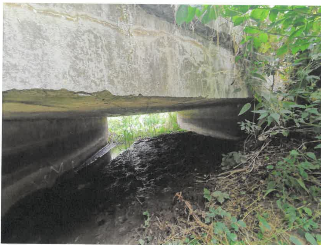
Fig.9 – Infiltratii la infrastructura
